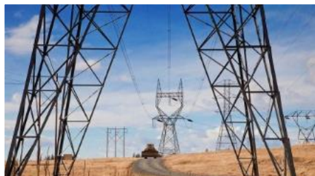
Transmission Up to 765kV
