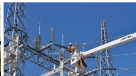
Substation Up to 765kV
