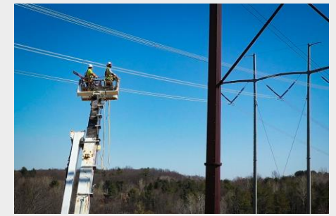
CENTRAL EAST ENERGY CONNECT New York; $300M+; 3 ½ year project Nearly 100 miles of 345kV transmission
