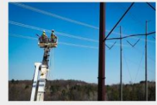
CENTRAL EAST ENERGY CONNECT New York; $300M+; 3 ½ year project Nearly 100 miles of 345kV transmission
