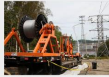
MAINE POWER RELIABILITY PROGRAM Maine; $200M+; 4-year project 210 miles of 345kV & 115kV transmission line
