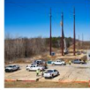
CENTRAL EAST ENERGY CONNECT New York; $300M+, 3.5-year project; nearly 100 miles of 345kV transmission
